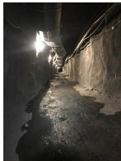
Figure 1-5 Ducting Inside of Tunnel
