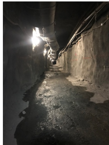
Figure 5 Ducting Inside of Tunnel
