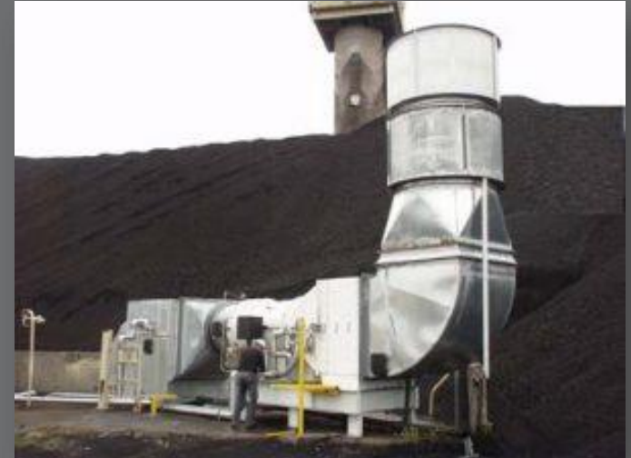
60,000 cfm T-46 Coal Reclaim Tunnel
